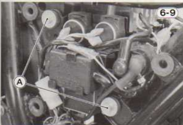
A. Electrical Panel Mounting Bolts
